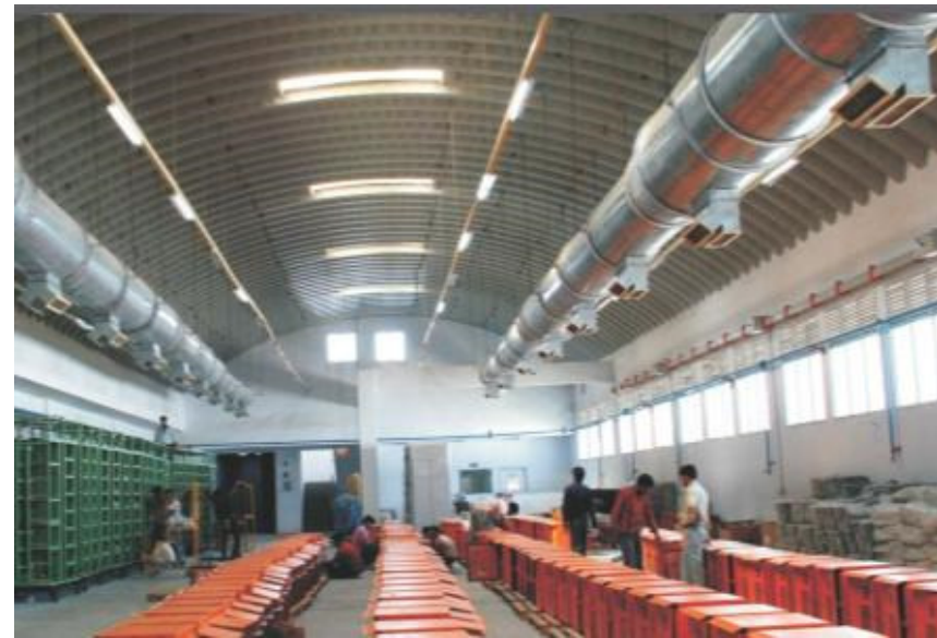
Ducts Hanged from the Roof
