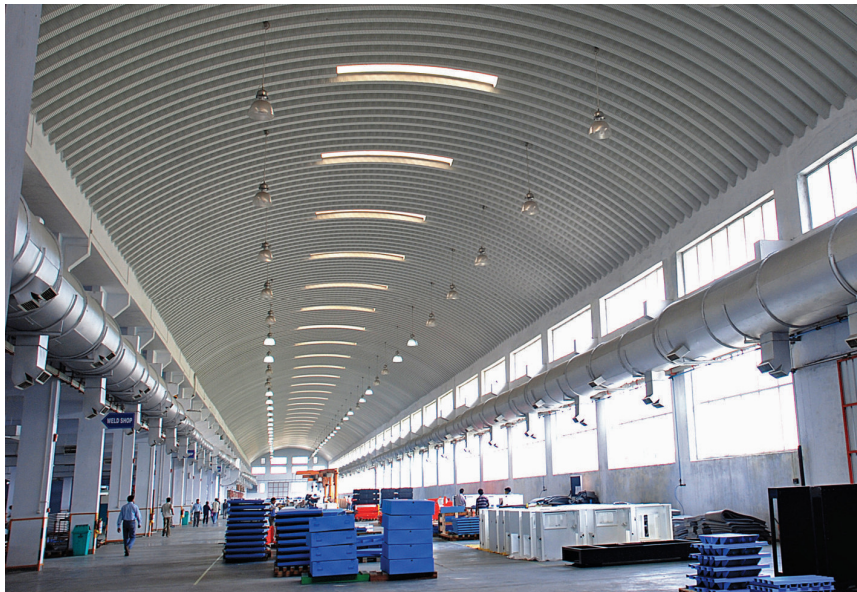
Hangers and Ducts
